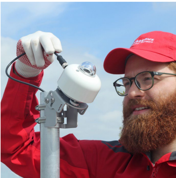
Figure 10 PMF01 pyranometer mounting fixture can be used for easy installation of a pyranometer in Plane of Array (POA) for PV system performance monitoring.
