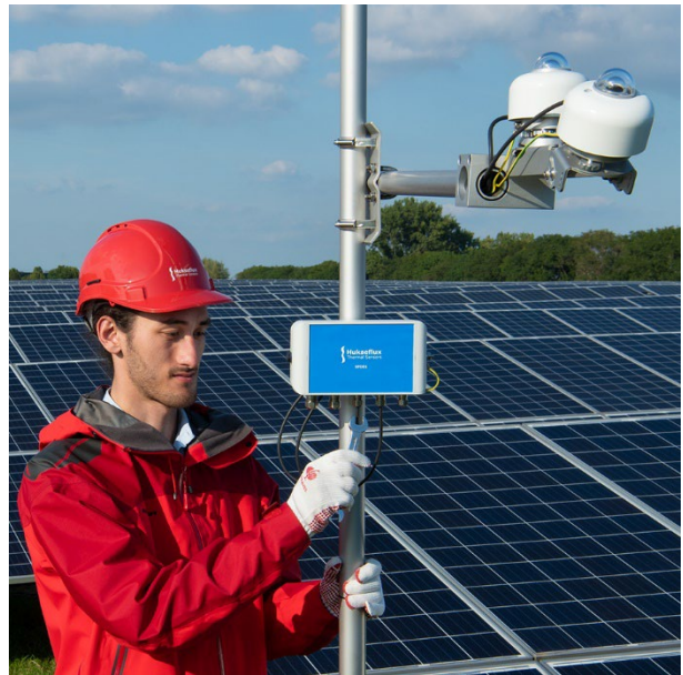
Figure 6 Two SR300-D1 pyranometers that are connected to the SPD01 Surge Protection Device. With the optional SPD01, you can upgrade surge immunity to Level 4.
