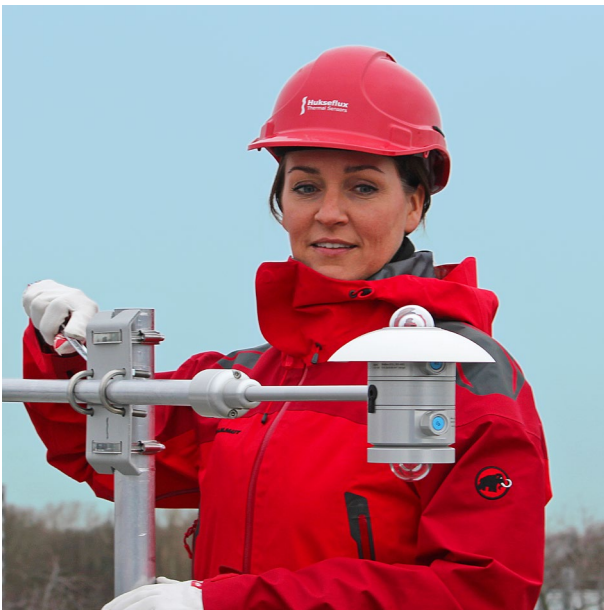
Figure 6 Installation of AMF02 albedometer mounting kit and two SR20 pyranometers, mounted with ALF01 leveling fixture on a crossarm with crossarm bracket CMF01.
