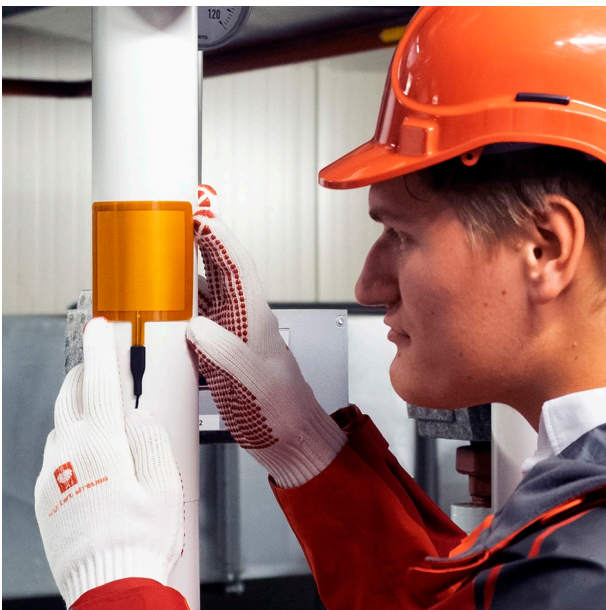
Figure 2 Model FHF05-85X85 heat flux sensor installed on a pipe.
