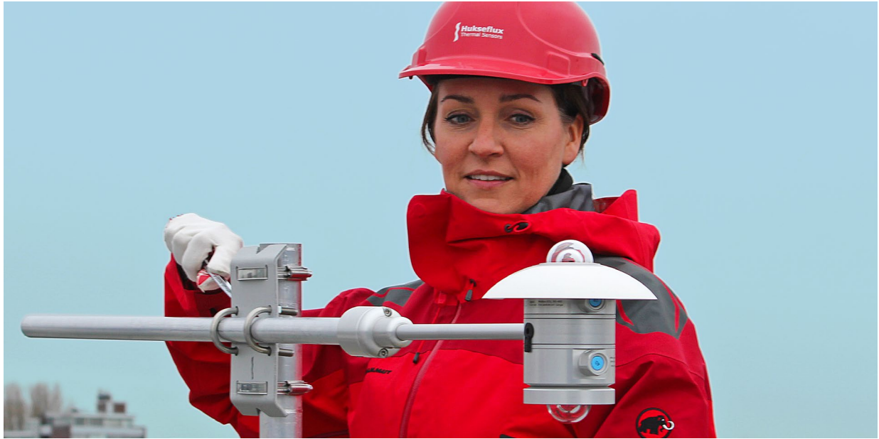
Figure 3.4.3 Installation of an albedometer mounted with AMF02 albedometer mounting fixture and levelled with ALF01 albedometer levelling fixture. The crossarm mounting fixture, connecting the cross arm to a vertical mast is CMF01
