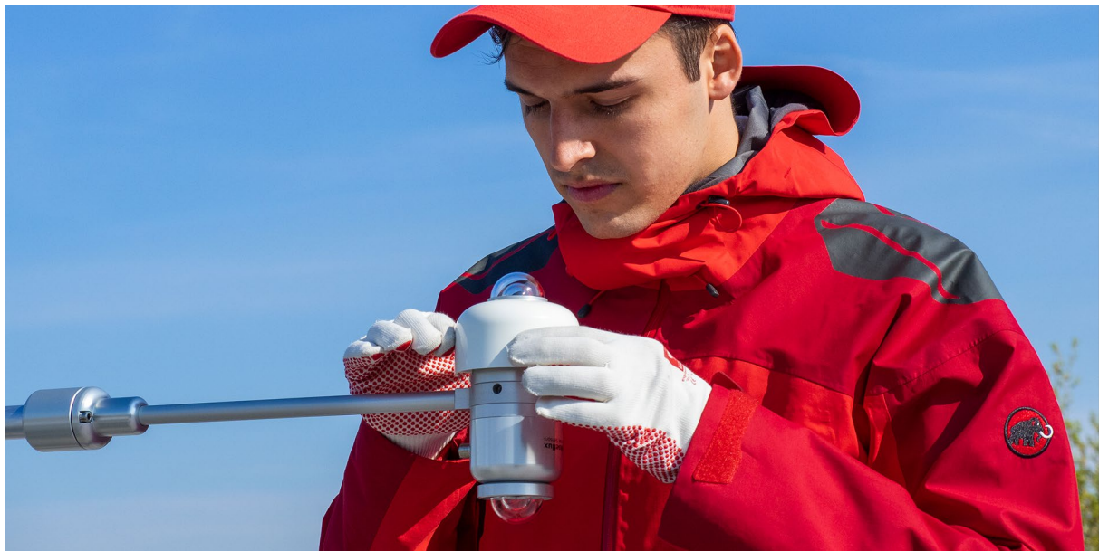
Figure 0.4 Installation with AMF03, two SR30-M2-D1 pyranometers and ALF01 levelling fixture
